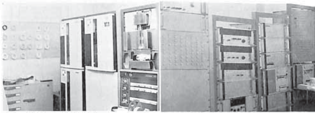
Photo. 1 1st DP Room (CPU and MT)
